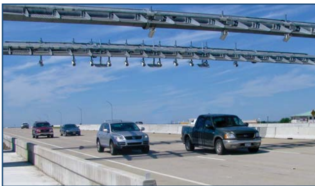
Electronic toll collection equipment at a toll gantry
